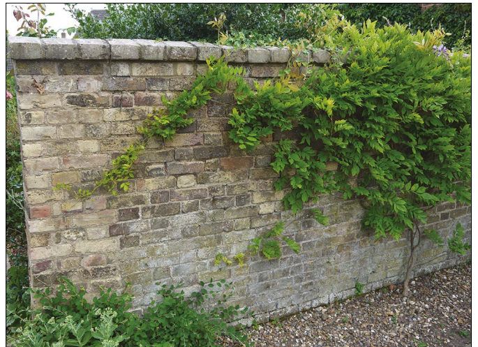
Figure 44: Lodge Close Wall.
